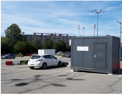
Air quality station «Plaines-du-Loup» Lausanne, Switzerland
