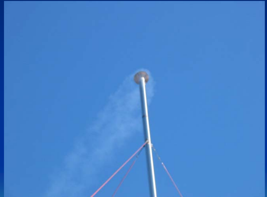
Engine Exhaust Stack
